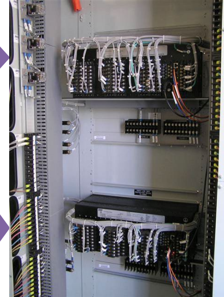
Integrated P&C system using fiber optic network cables
